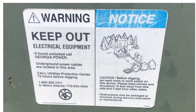
Fig 8: Signage on electrical box outside the fence line, indicating the presence of underground electrical wires which, in the absence of overhead wires, presumably provide the connection between the array and the grid.
