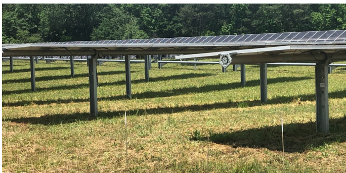
Fig 6: SAST- diagonal view. Small shadows directly beneath the modules, along with a very low rotational angle (modules pointing almost directly upwards) indicate the photograph was taken close to solar noon. Wider spacing between rows (compared to fixed-angle arrays) is visible. In early morning or late evening, modules will be rotated at steep angles, casting shadows up to the adjacent rows.
