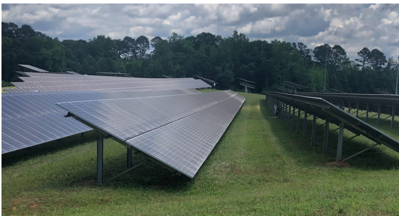
Fig 4. Along-row view of Array C/D demonstrating tightly-packed rows (high Ground Coverage Ratio, GCR) with minimal space require between rows to prevent mutual-shading. The PV supporting structures are clearly seen to be rigid, with no mechanical equipment. The resulting lower overall weight allows for simpler siting in the ground. Electrical equipment connecting module rows into the larger array are placed under the module rows, in shadow, to keep them as cool as possible for the sake of efficiency.
