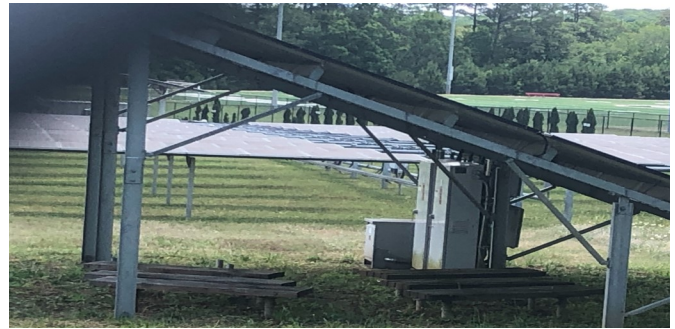
Fig 5. View of electrical equipment (presumably batteries) under the shading of Array F, fixed axis, facing south.
